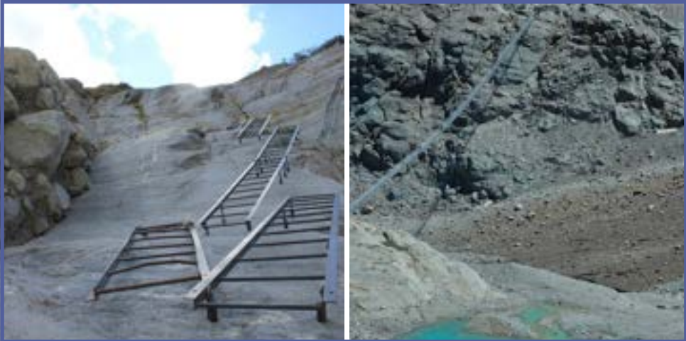
Figure 21. Maintaining access to high mountain huts through the installation of equipment: a challenging construction project. Left: 90 meters of ladders connect the Montenvers train to the Mer de Glace (photo: J Mourey). Right: a 190-meter suspension bridge above the toe of the Corbassière Glacier (Valais, Switzerland) to allow access to the Panossière cabin (2,641 m; photo: J.-L. Pitteloud).
